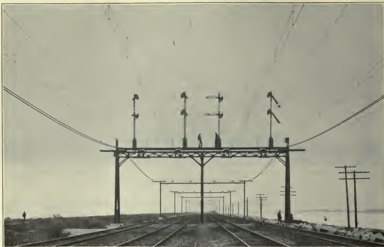
FIG. 527. OVERHEAD CONTACT SYSTEMS. Catenary Construction, 1,200-Volt Direct Current Main Line, Southern Pacific Railroad, near Oakland, Cal.
